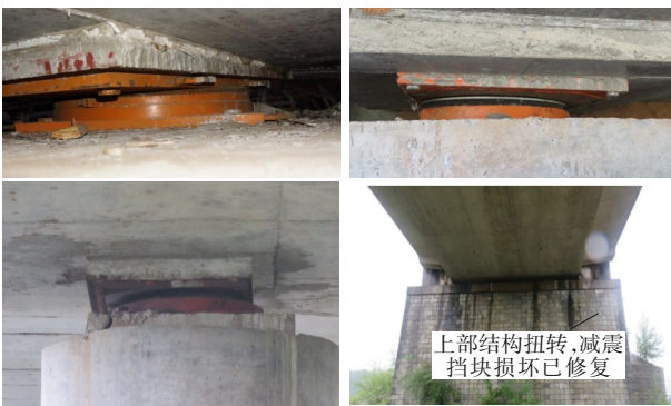
图2 上部结构扭转超出支座滑动范围导致减震挡块破损 Figure 2 Damage to seismic arrestor resulting from torsion in superstructure exceeding bearing's sliding range
